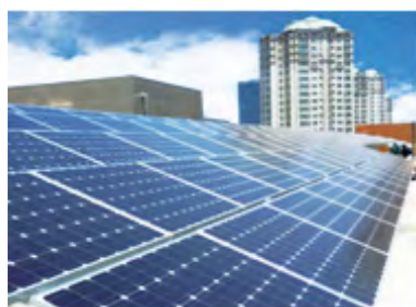
Solar Energy Power Plant
