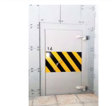
Blast proof doors
