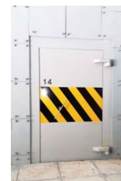
Blast proof doors
